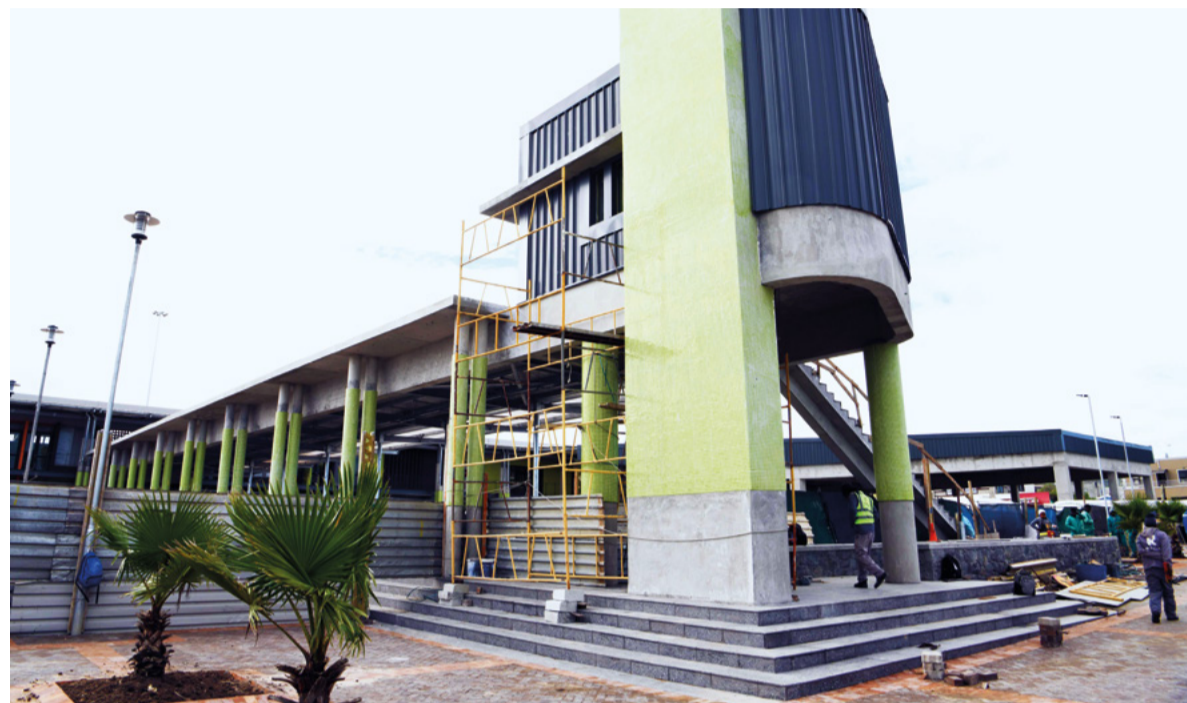
Travel treasure: The City has completed the upgrade of the Dunoon public transport interchange (PTI). Construction of the multi-storey building, a covered waiting area for commuters and public open spaces started in 2019. There are ablution facilities and formal trading kiosks, as well as outside informal trading spaces to stimulate economic development.
